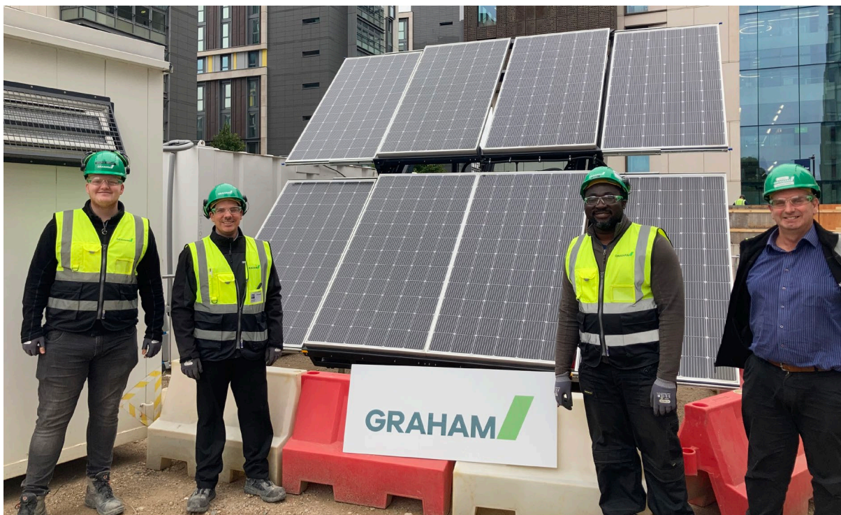
Figure 3 – Solar Hybrid Generator in use at School of Public Health, Imperial College London, White City Campus
